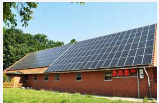
37.4 kWp with MAGE POWERTEC® PLUS modules Lünne, Germany
